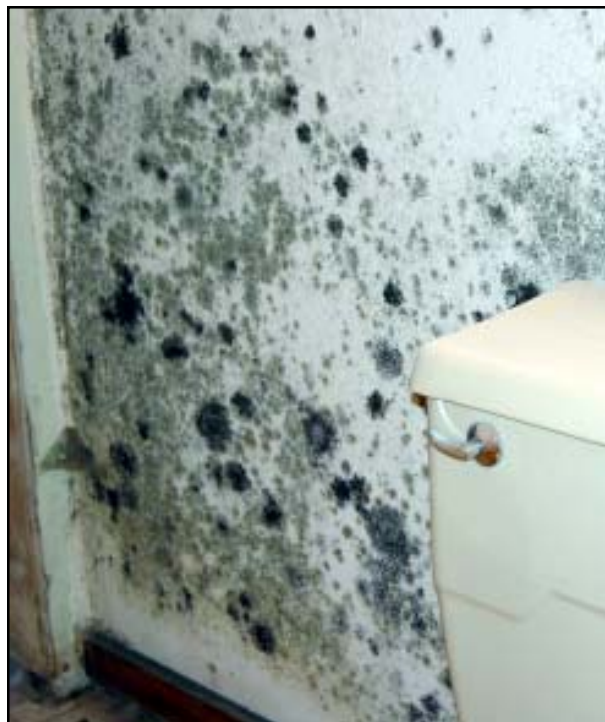
Many mold colonies growing on dry wall in a residence. (Image courtesy of Dr. Chin S. Yang of P&K Microbiology Services)
