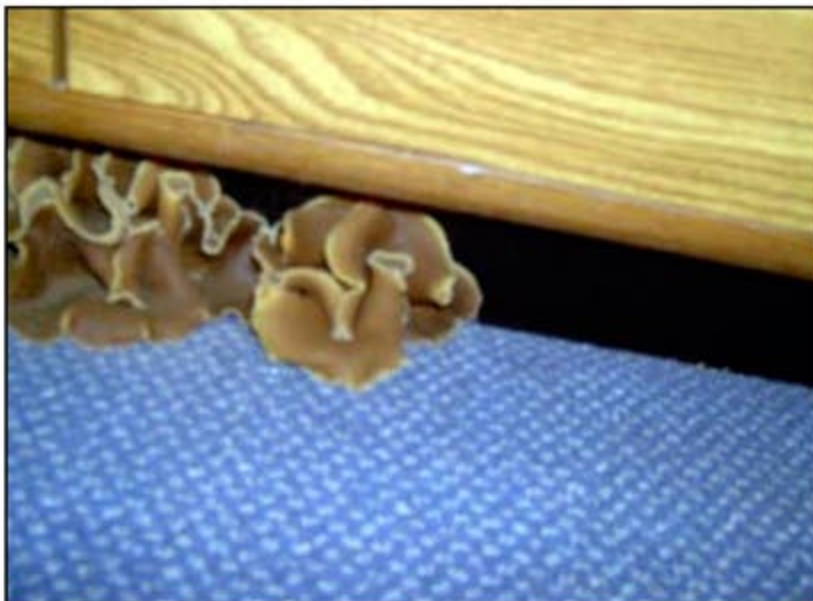
Fruiting bodies of a Peziza sp. in a room with chronic water damage. Peziza sp. is an ascomycete (producing sexual ascospores in a structure called the ascus) and is also known as one of the cup fungi. It is occasionally found on chronically wet or water-damaged wood products (such as plywood subfloor). Peziza can be identified only when the sexual fruiting body is present. In culture, its vegetative state is named Chromelosporium sp. (Image courtesy of Michael Underhill, CIH, CSP of Trident Environmental Services, Inc.)
